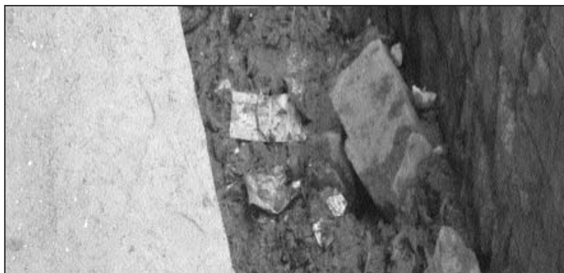
An open drain at Kamraj Road
