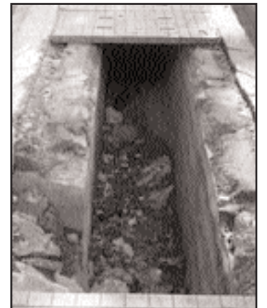
Missing slabs expose drain
